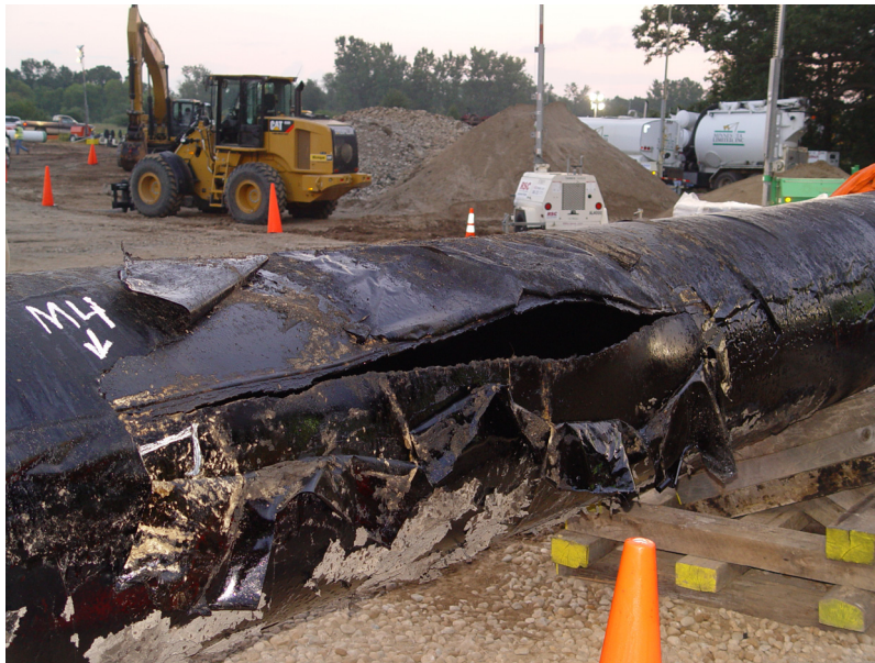
Enbridge Line 6B ruptured near Marshall, Michigan, June 2010. Source: National Transportation Safety Board
